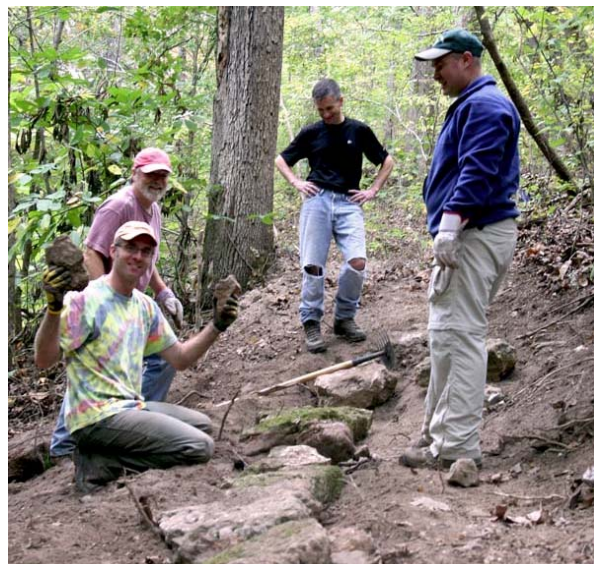
Digging a trench for rocks to keep soil on the trail (l-r): Joel Luedders, Frank Wentz, John Brett and Todd Horn (Crew Leader) on the Oct. 13, 2007 North Courtois Outing
